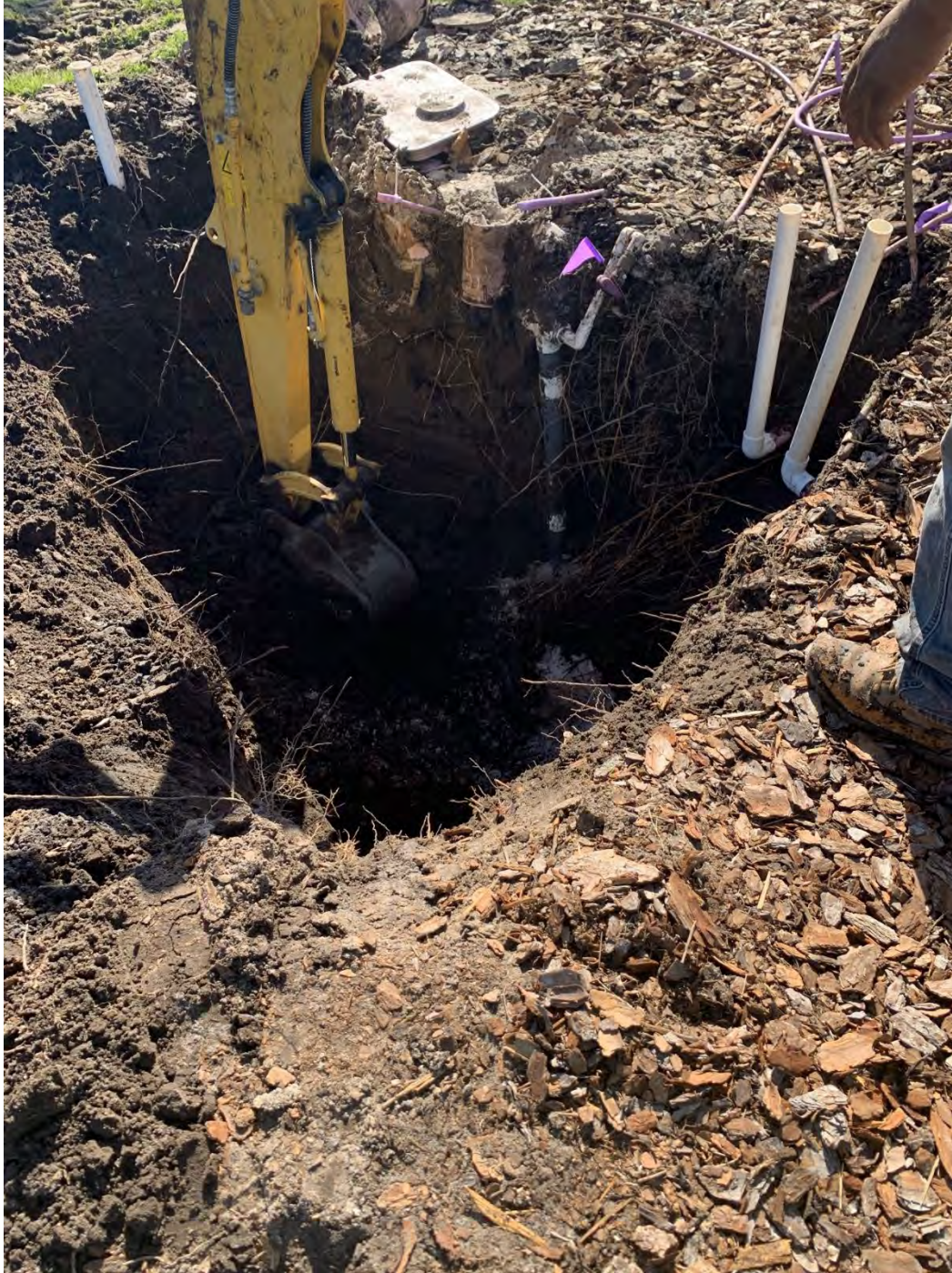
8' deep hole required to repair mainline leak in center island of Watterset Blvd., south of Milestone.
