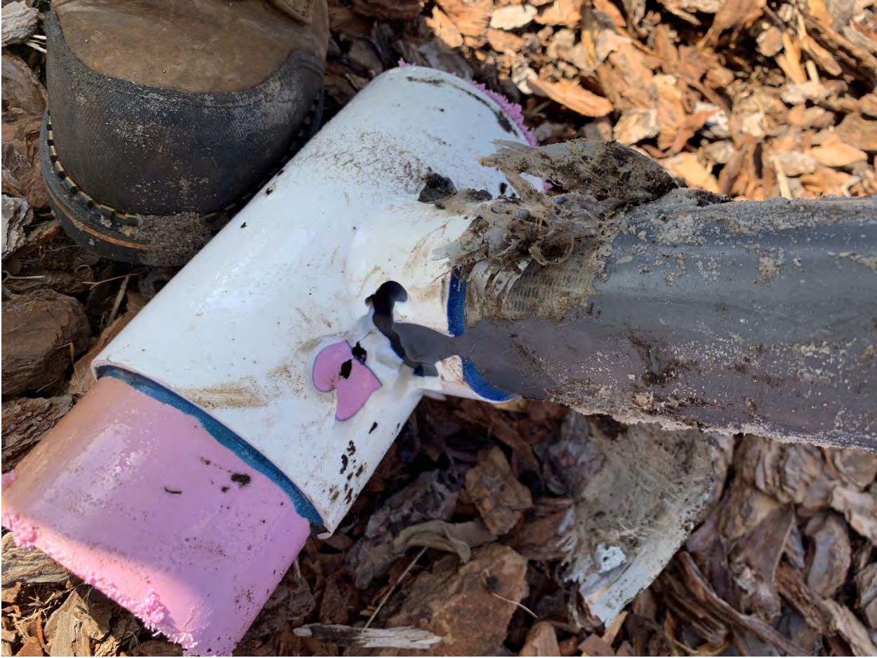
Damaged fitting causing leak in center island of Wasset Blvd., south of Milestone.
